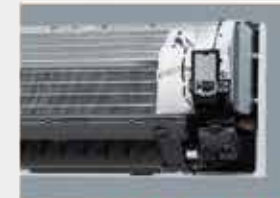
Ensure its reliable operation and preventing fire accident in case of short circuit.
